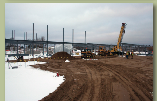
Pictured: Construction begins on the Community & Government Services Facility. Photos courtesy of Bois Forte Communications.
